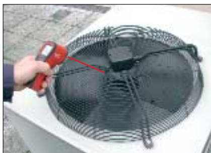
Safely diagnosing the status of a system by measuring the temperature of safety valves, pumps and other wearing parts.
