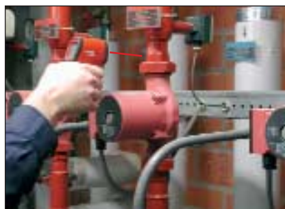
Checking supply and return flow to help determine efficiency of heating / cooling systems in seconds, not minutes.
